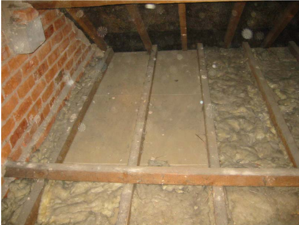
Photo 1. Existing fibreglass insulation was missing to a large area. This was not visible from a head and shoulders inspection of the roof space. Note fibres in air caught by camera flash.
