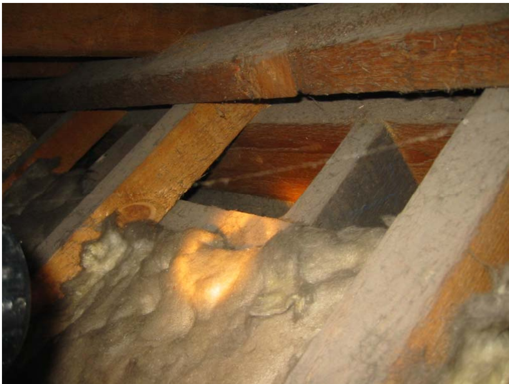
Photo 2. Edges of roof space not insulated.
